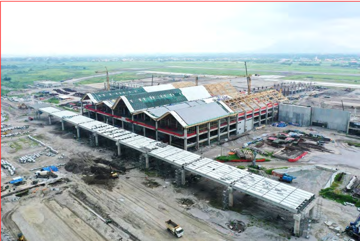
Figure 6: Installation of steel decking and Girder installation substantially completed in Elevated Road.
