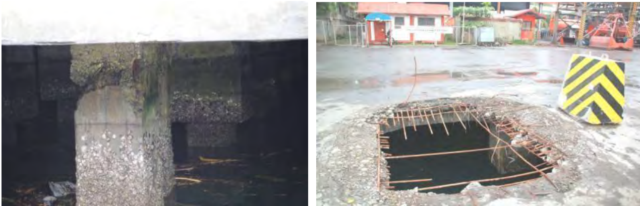
Figure 7 and 8: Existing pile head and Damaged Portion of R.C. Deck (Old Pier) (Source: HPC 2013)
